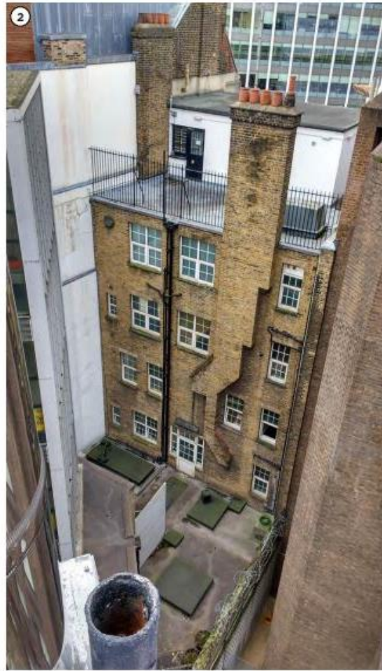
2. View of the rear of the Snow Hill block (Block 'A') and view of the link building between the blocks.
